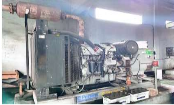
Figure 1. Generator Capacity 500 kVA
