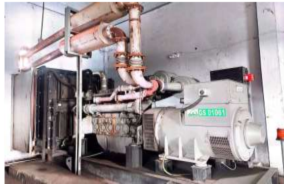
Figure 2. Generator Capacity 800 kVA
