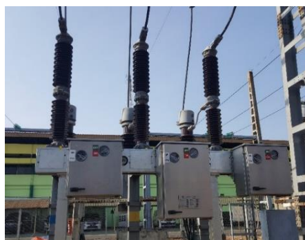
Figure 9. PMT Baru Bay Kuningan II Merk UNINDO.
